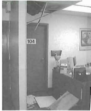
Before (leaking roof damage)
